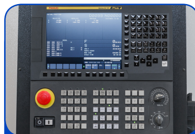
PAINEL OPERACIONAL FANUC
